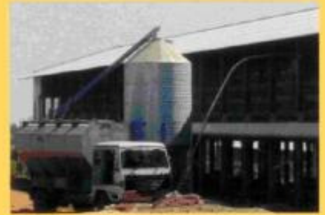
Feed Silo and Conveyors
