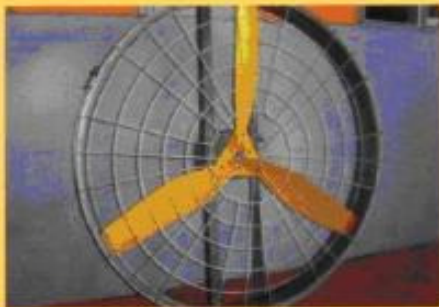
Air circulating fans
